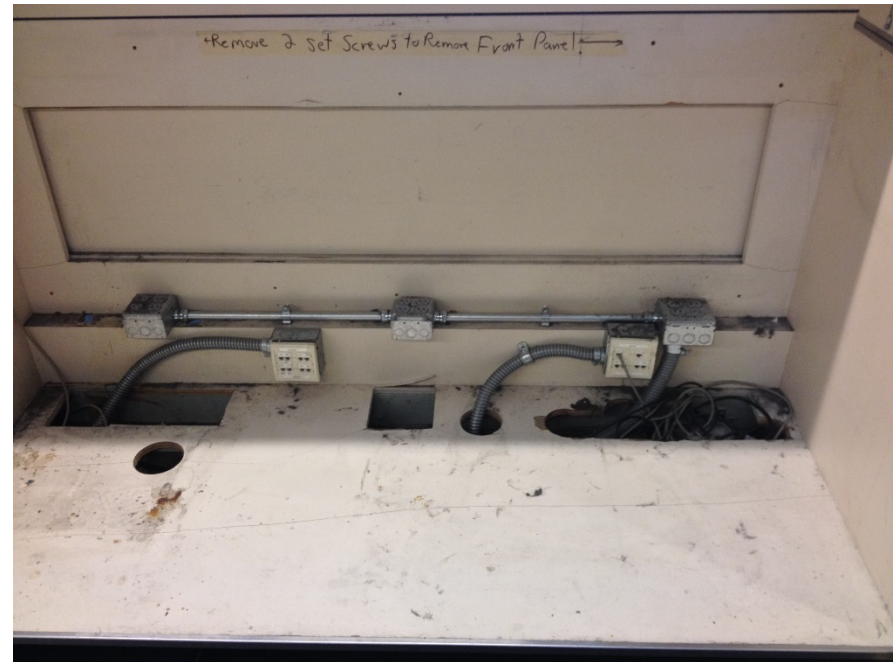
Figure 12 – Power and Comm Cabling to a Typical Counter Shell
