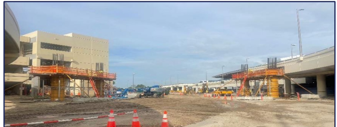
Roadway Improvements – Forming and Internal Reinforcement for Ped Bridge & Columns *as of 5.28.26
