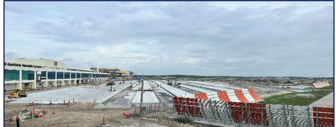
Airside Improvements– North side of Concourse E Concrete Pavement for Commercial Apron *as of 5.28.26
