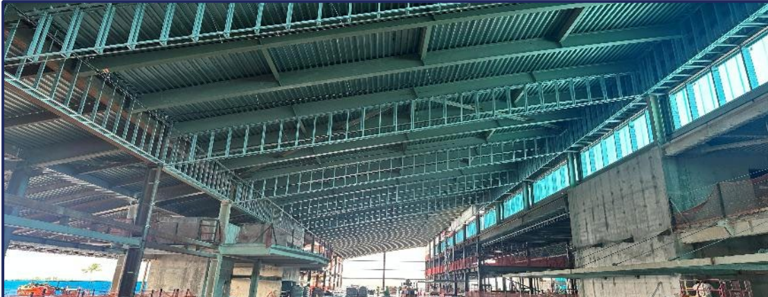
Main Terminal – Departures facing west by Zone 22 & 23 Light Gauge Metal Framing & Curtainwall *as of 5.28.26
