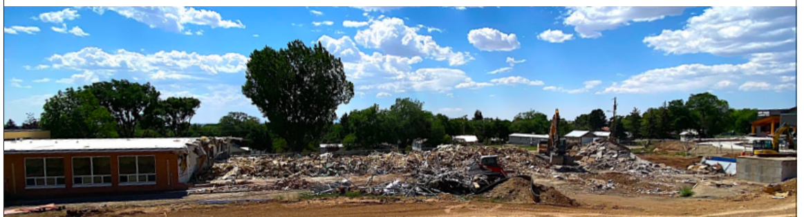
7th Street Elementary was finally torn down completely, part of the grounds will be rebuilt into playground and parking areas.
