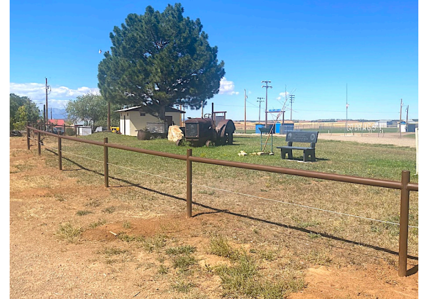
Dove Creek Recreation Dept - Weber Park upgrade new metal fencing will last for many years to come.
